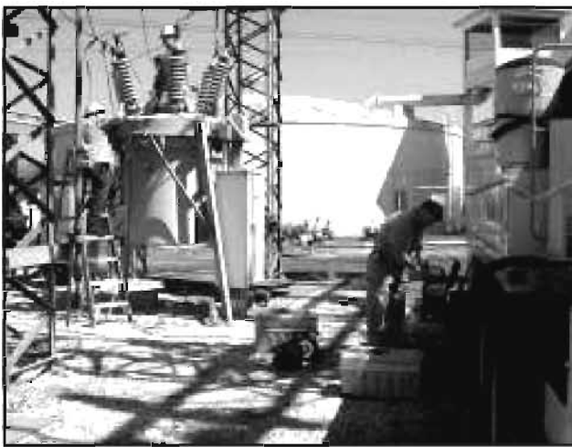
Figure 27: DF of OIP 66kV bushings (aged)
